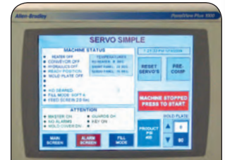
AB Touchscreen Controls
