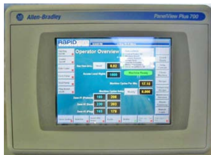
Allen Bradley PanelView Plus Touchscreen
