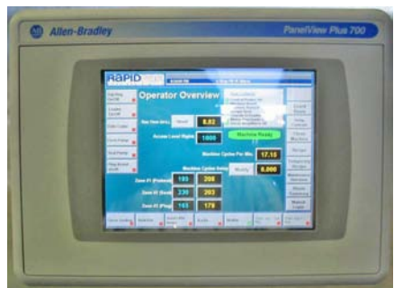
Allen Bradley PanelView Plus Touchscreen
